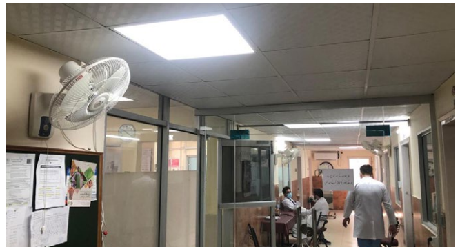
Picture 8: Replacement LED panels in the gynaecology ward
