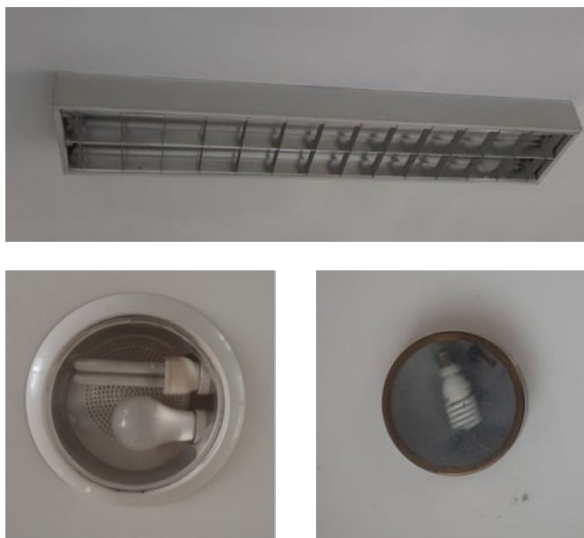
Picture 2. Surface mounted fluorescent tube luminaire and downlight luminaires at NEECA building
