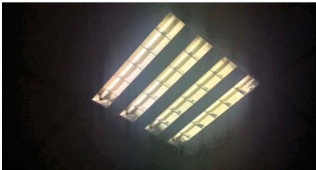
Picture 7. Surface mounted fluorescent tube luminaire
